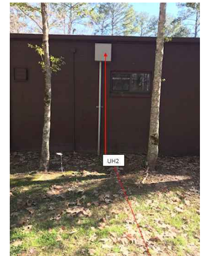
@ 15+12 PLACE 3/4" CONDUIT FROM UH-2 UP THE WALL. MAKE SURE CONDUIT IS FLUSH WITH WALL.
